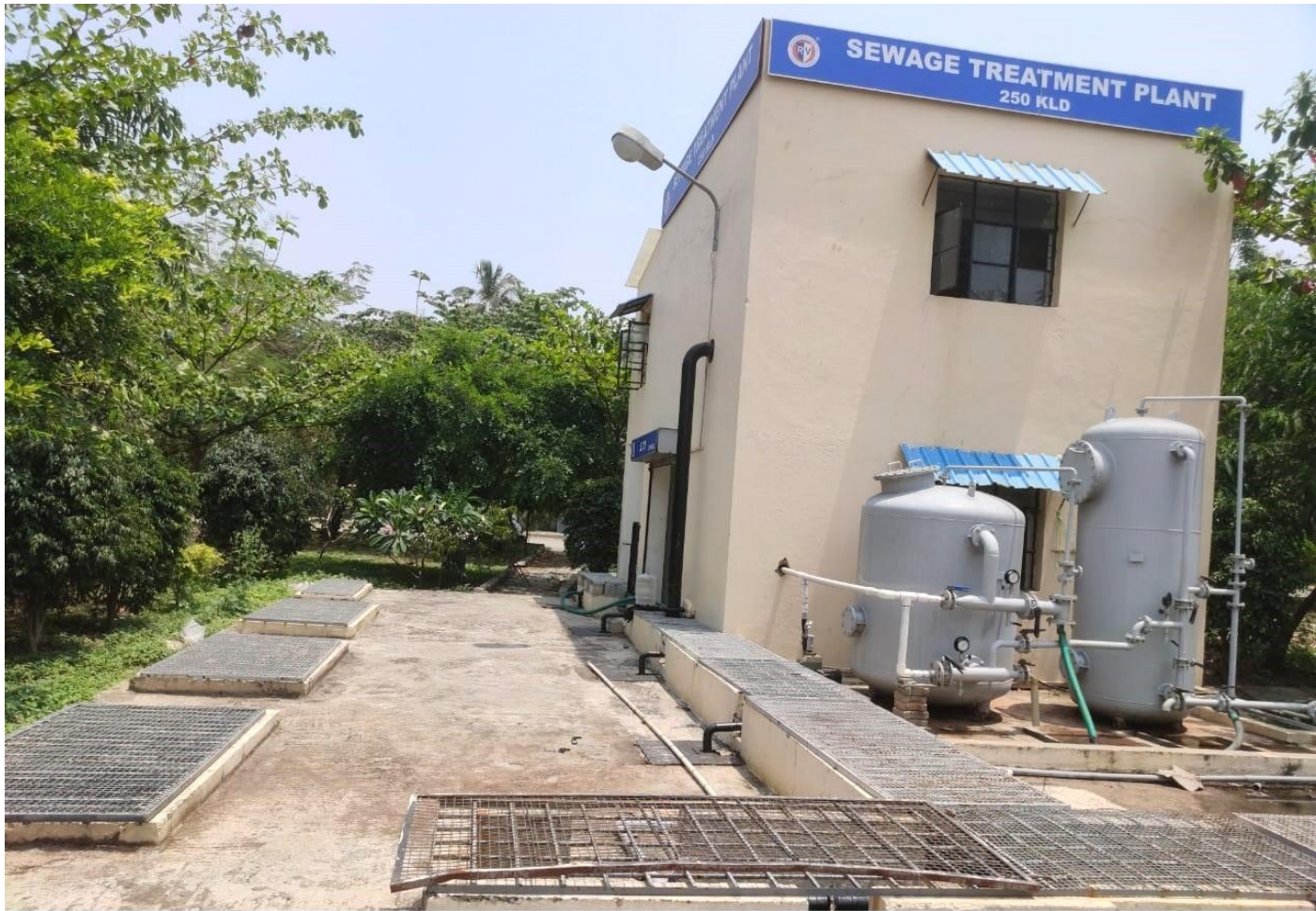
Sewage Treatment Plant: 250KLD
