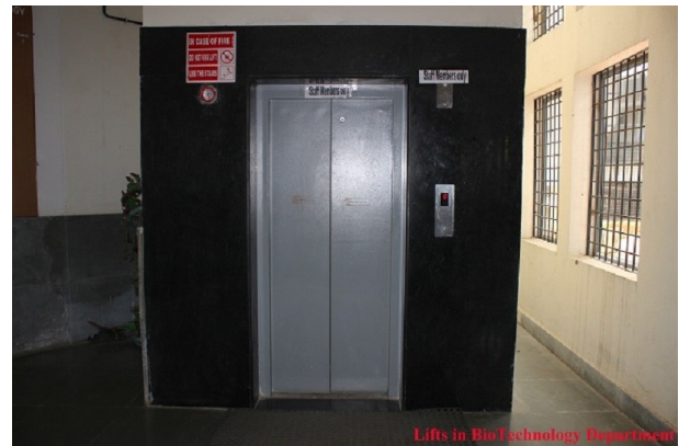
Lifts in BioTechnology Department
