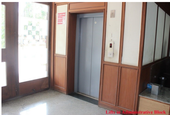
Lifts in Administrative Block
